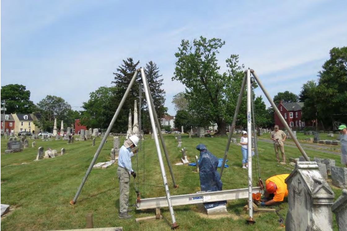
Two I-Beam Hoists Attached to I-Beam Ends with C-Clamp Stops & Main Hoist Attached to Trolley
