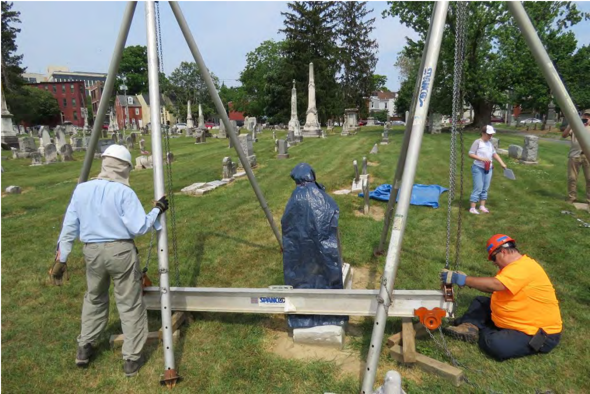
Trolley and One End Hoist attached to I-Beam with Level Attached to Center of I-Beam
