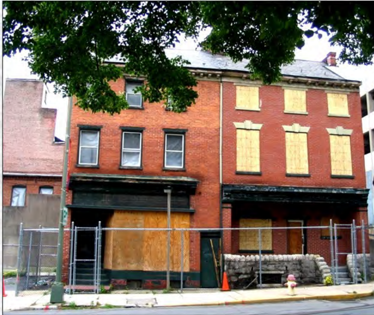
23 East Vine Street (right) undergoing rehabilitation, 2006 After Stevens' death, she acquired adjoining land and built 21 East Vine Street (left).
